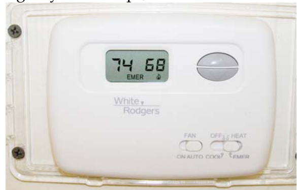
Emergency Heat Strips, Switch Set to Position 4
